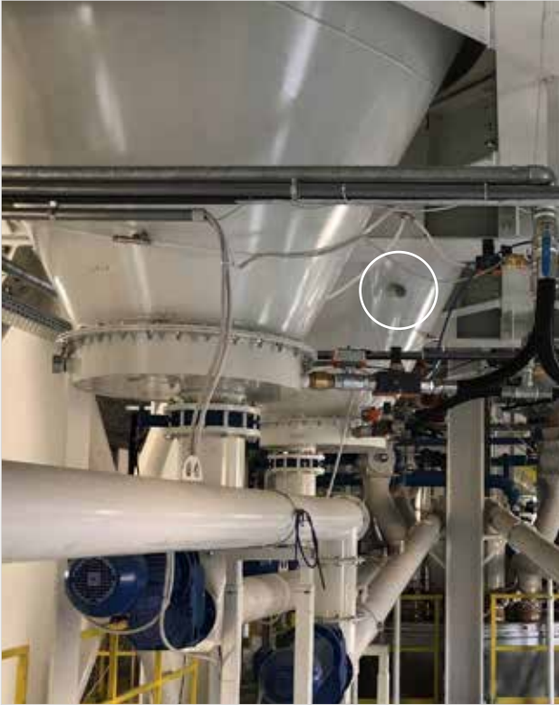
VBS (aerators) - Silos
